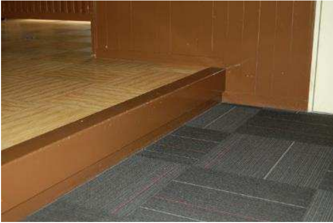
Changing room entrance: There are some gaps, (no slopes)
